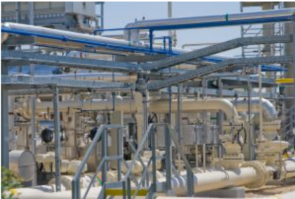
Natural gas infrastructure
