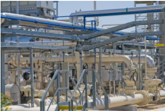
Natural gas infrastructure
