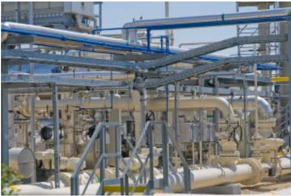
Natural gas infrastructure
