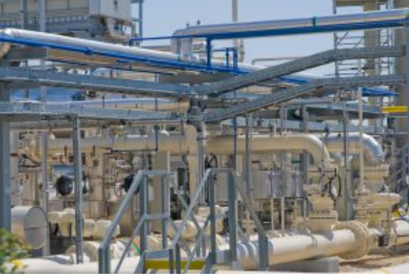
Natural gas infrastructure
